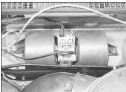
20.6 Heater motor and wiring
